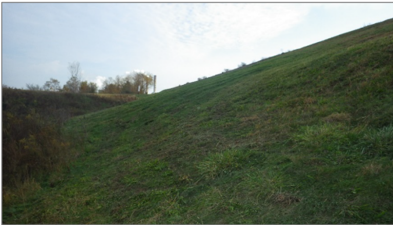
Photo 32, Point 31 Northwest Exterior Slope – Bare spot on the slope near mid- height.
