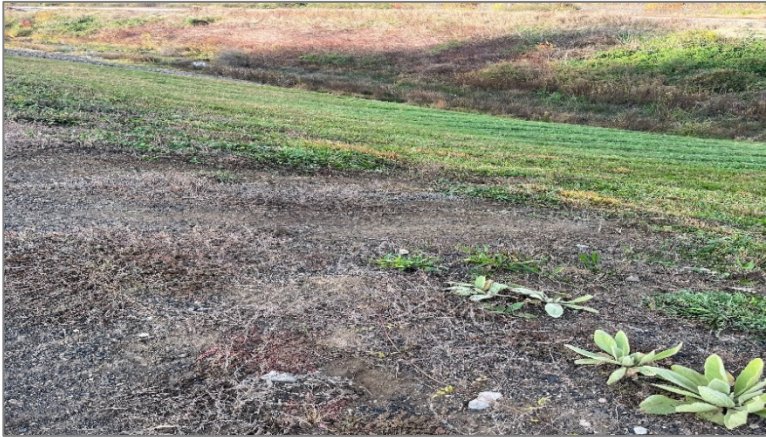
Photo 25, Point 24 Northwest Exterior Slope – Bare spot near the crest.
