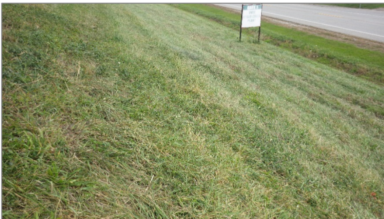
Photo 39, Point 38 Southeast Exterior Slope – Bow in the slope at mid-height.
