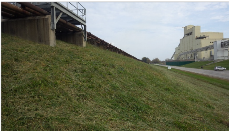
Photo 36, Point 35 Southeast Exterior Slope – Depression at mid-height of the slope.
