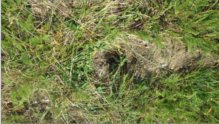
Photo 10, Point 10 Boiler Slag Pond – Southeast Exterior Slope – Animal burrow near the toe.
