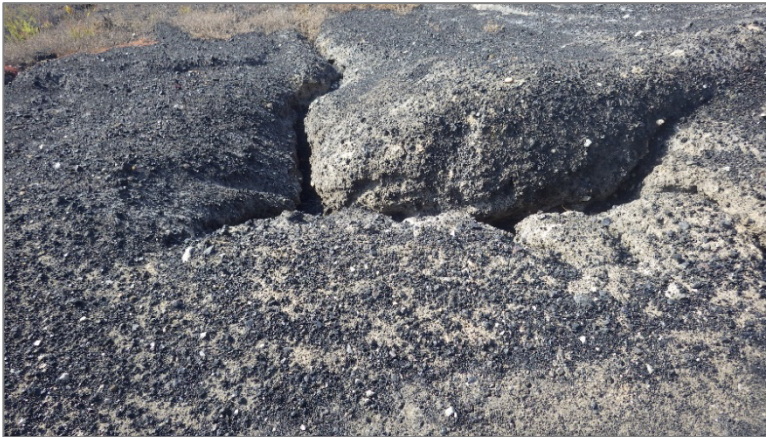
Photo 13, Point 13 Boiler Slag Pond – Southwest Divider Dike – Erosion gully at the crest.
