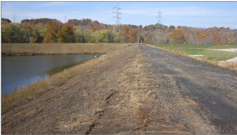
Photo 11, Point 11 Boiler Slag Pond – Southwest Divider Dike – Erosion gully and rutting in exterior slope.
