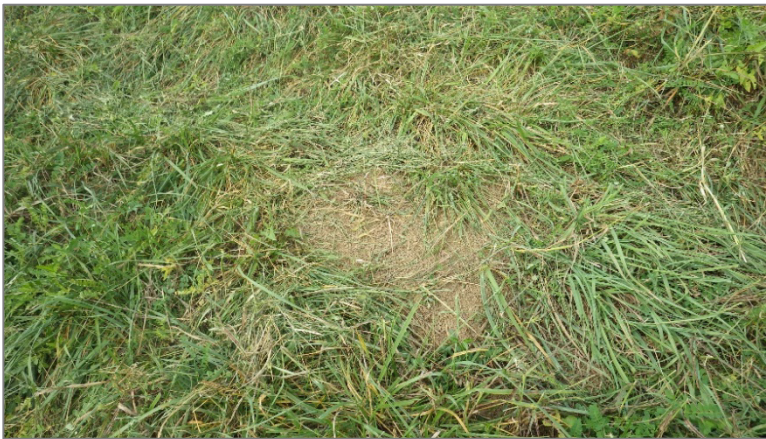
Photo 44, Point 43 Northeast Exterior Slope – Animal burrow near the toe.
