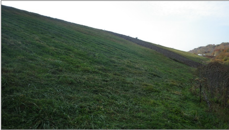
Photo 28, Point 27 Northwest Exterior Slope – Depression in lower half of slope.
