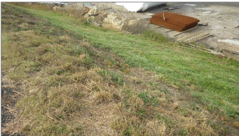
Photo 33, Point 32 West Exterior Slope – Bare spot on slope near the crest.
