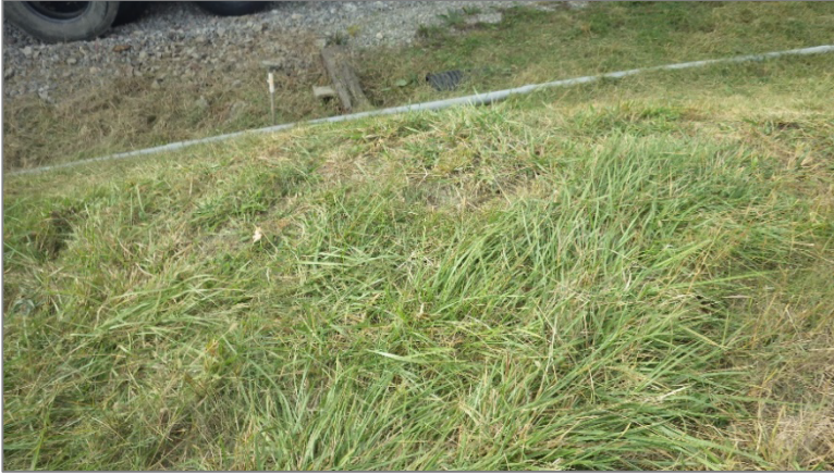
Photo 46, Point 45 Southwest Exterior Slope – Slough on slope.
