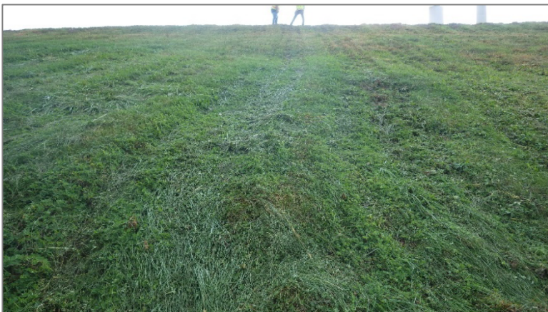
Photo 30, Point 29 Northwest Exterior Slope – Depression in lower half of slope.
