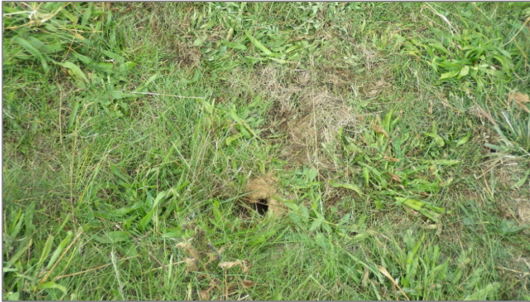
Photo 31, Point 30 Northwest Exterior Slope – Animal burrow near the toe.
