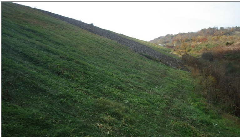
Photo 29, Point 28 Northwest Exterior Slope – Depression in lower half of slope.
