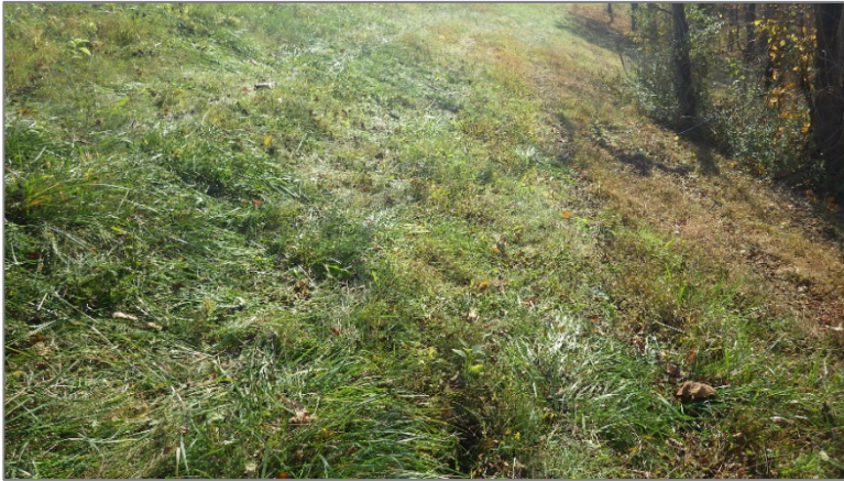
Photo 16, Point 16 Boiler Slag Pond – West Exterior Slope – Erosion gully near the crest.
