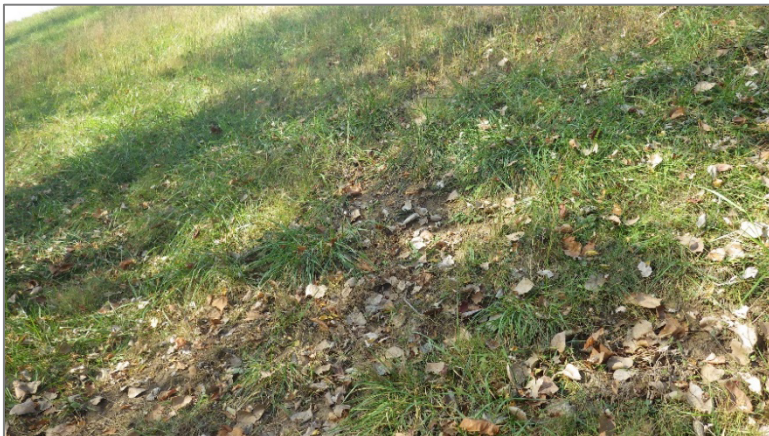
Photo 2, Point 2 Boiler Slag Pond – Southeast Exterior Slope – Erosion gully near the crest.
