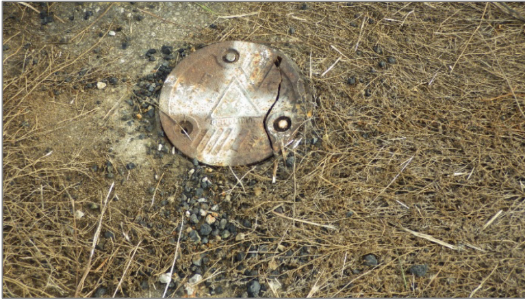
Photo 34, Point 33 West Exterior Slope – Damaged well lid on instrumentation.
