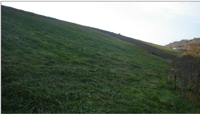
Photo 26, Point 25 Northwest Exterior Slope – Depression in lower half of slope.
